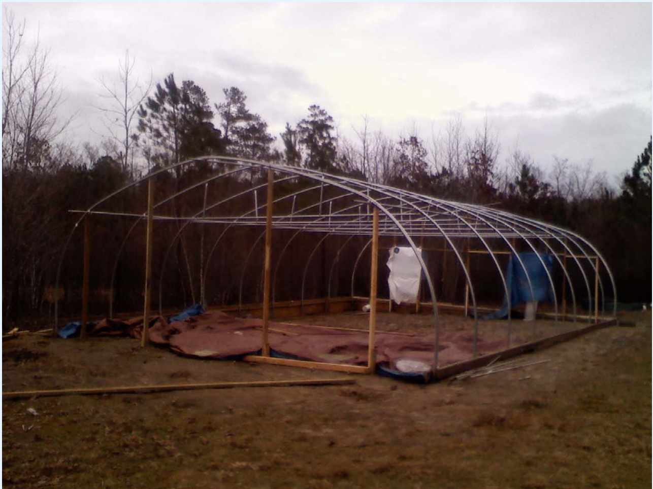
GREENHOUSE #2 IN THE MIDST OF RE-ASSEMBLY AT GROW AND SHARE DONATED SITE
